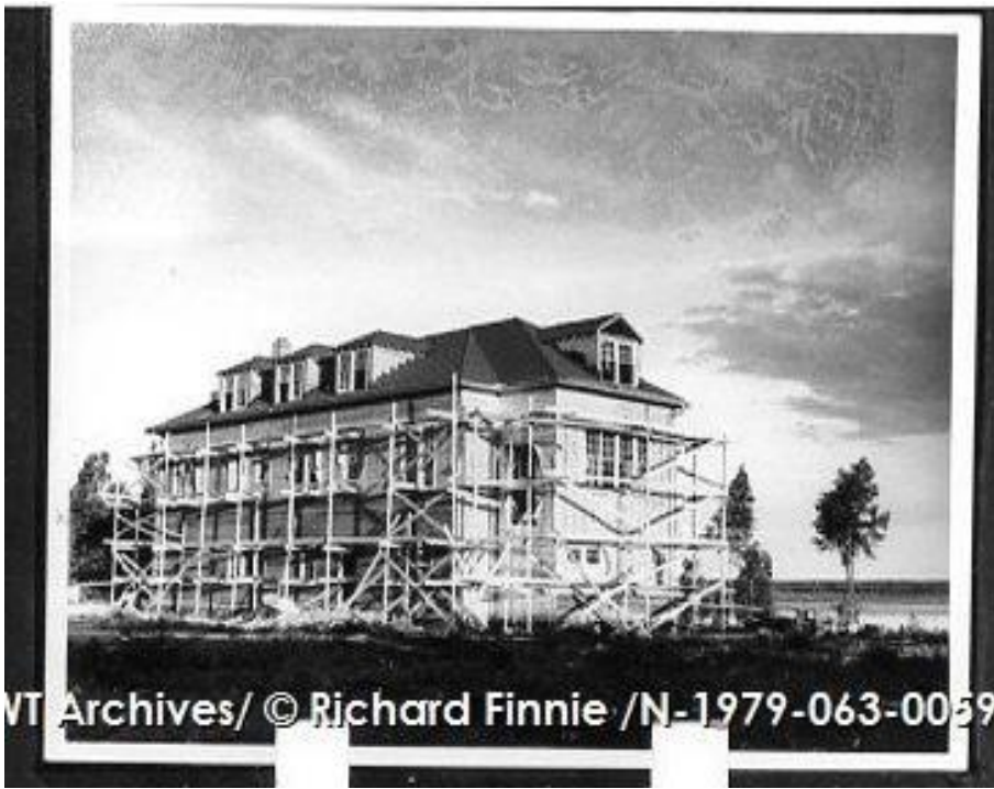
Fort Norman, 1939, Bishop Sovereign Anglican Hospital under construction at Fort Norman. It was destroyed by fire only two years later. Photo by Richard Finnie.
